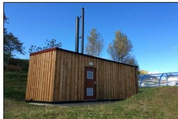
Biomass Boiler installation at Ardrishaig Primary School
