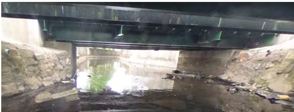
Figure 3.3 Underside of the Soroba Lane vehicle bridge, viewed from upstream looking downstream
