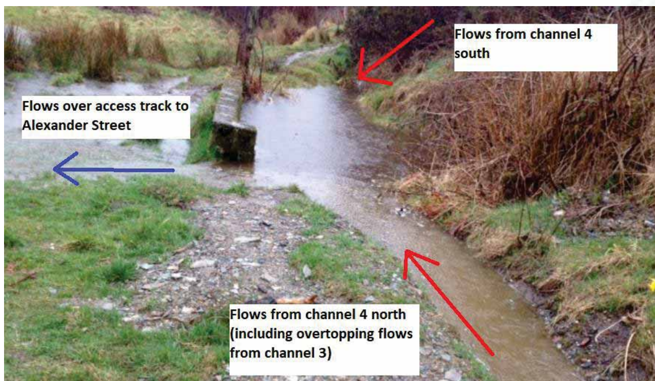
Figure 2-8: Channel 4 flooding mechanism at headwall due to under capacity/blocked culvert
