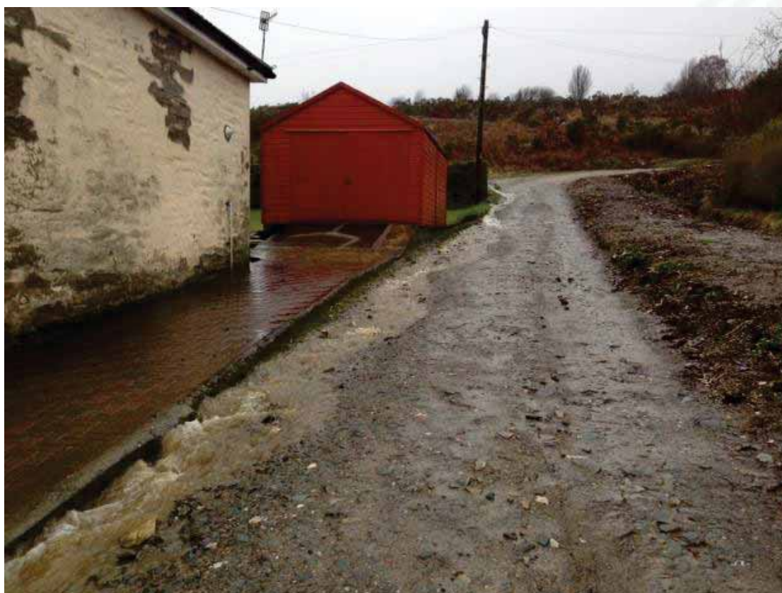
Figure 2-9: Channel 4 overflow down access track from confluence headwall
