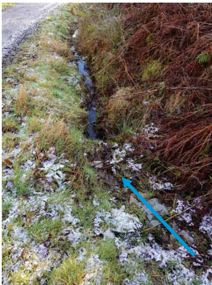
Figure 2-5: Point of overflow into Channel 4 north from over topping headwall of Channel 3
