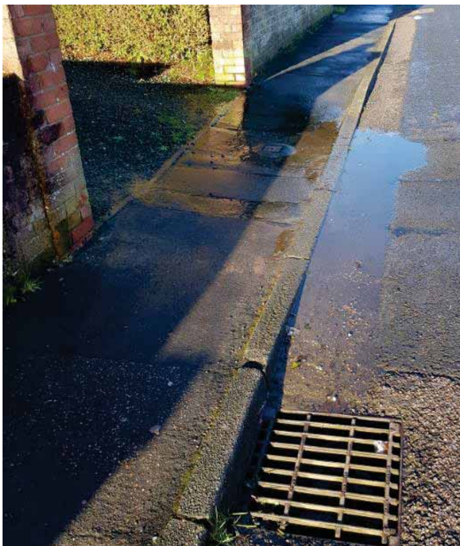
Figure 2-20: Ground water seepage emerging from gardens and driveways typical of properties along Alexander Street
