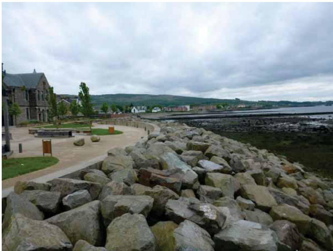
Figure 4-40: Photograph of defence within section S
