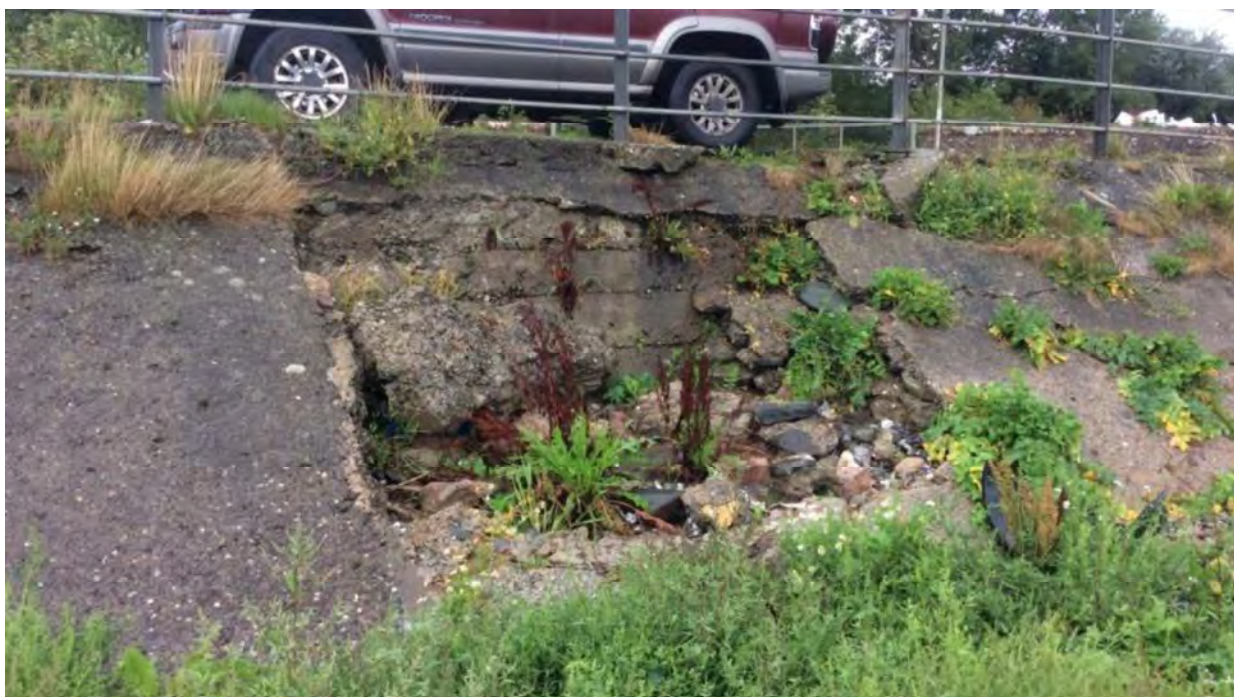
Figure 5-1: An example of failure of concrete revetment face at Craigendoran.
