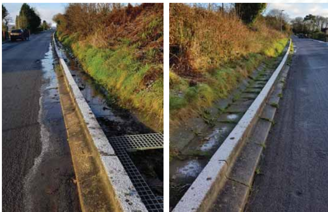
Figure 2-11: ABC installed drainage channel looking west from catch pit (left picture) and east from catch pit (right picture)
