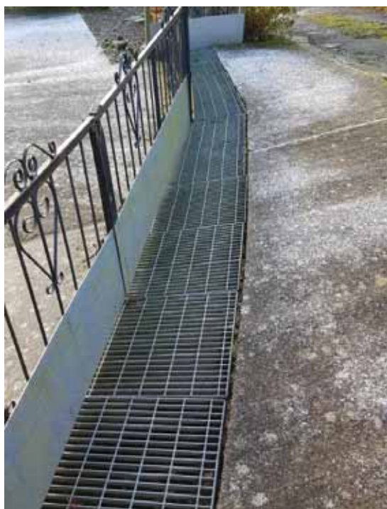
Figure 2-21: Drainage channel within property boundary to intercept flows and discharge back onto Tigh Dearg Road
