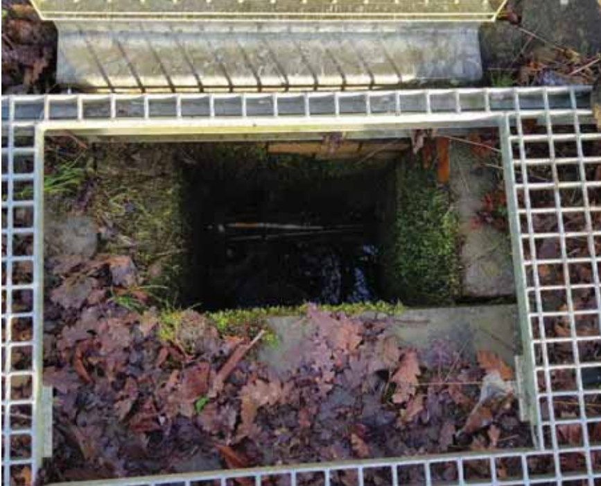
Figure 2-12: ABC installed catch pit with incoming flow from the hillside to the north discharging into the 225mm \emptyset combined sewer
