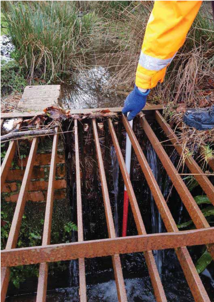
Figure 2-4: The headwall/chamber at which the watercourse west of Sandhaven (shown as inlet 4 on drawing No. 102740-003-DRG-9600-0B, Grontmij, 2010 – See Appendix B) enters the surface water network is blocked by upto 1m of silt and debris which should be removed to allow that channel to flow freely and reduce flood risk (this does not affect the properties in the north east of Sandhaven)
