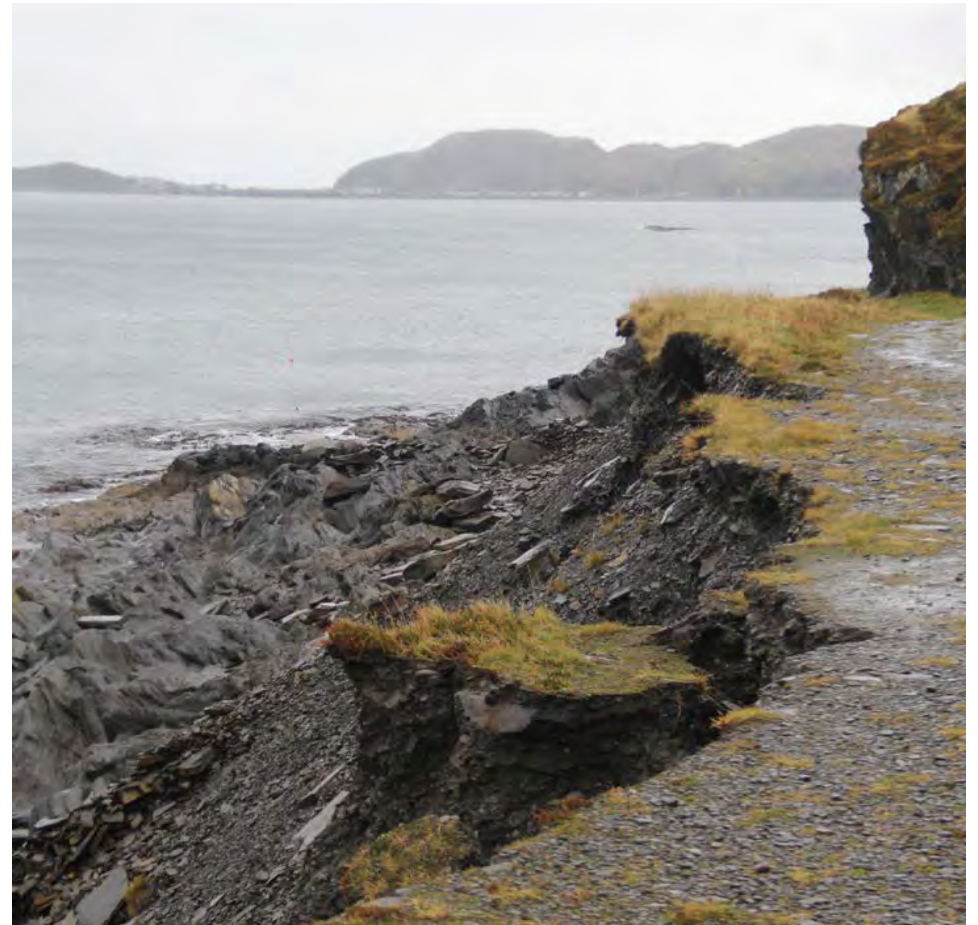
Coastal erosion to North of Cullipool
