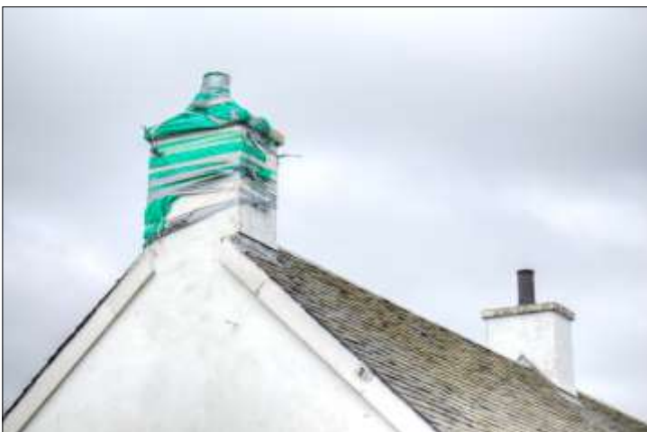
Chimney requiring maintenance
